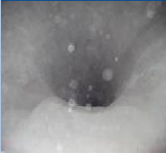
Plugged chute before Self-Cleaning liner
