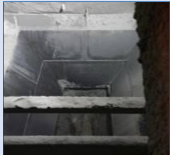
Clear chute after Self-Cleaning liner
