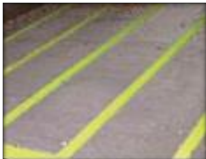
After: The woven wire screen was replaced with non-woven, self-cleaning screen cloth. This photo shows the panel one week after installation, with the pegging problem - and the need for frequent shutdowns - eliminated.
