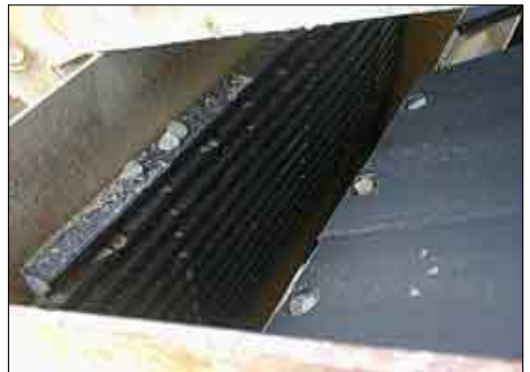
Screen discharge chute
